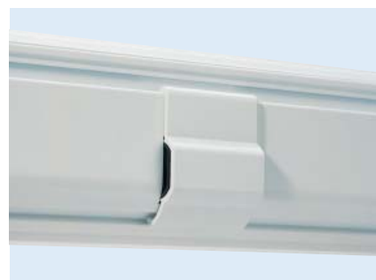
Electronic transformer (top) and wiring are hidden in the back wall of the casing
